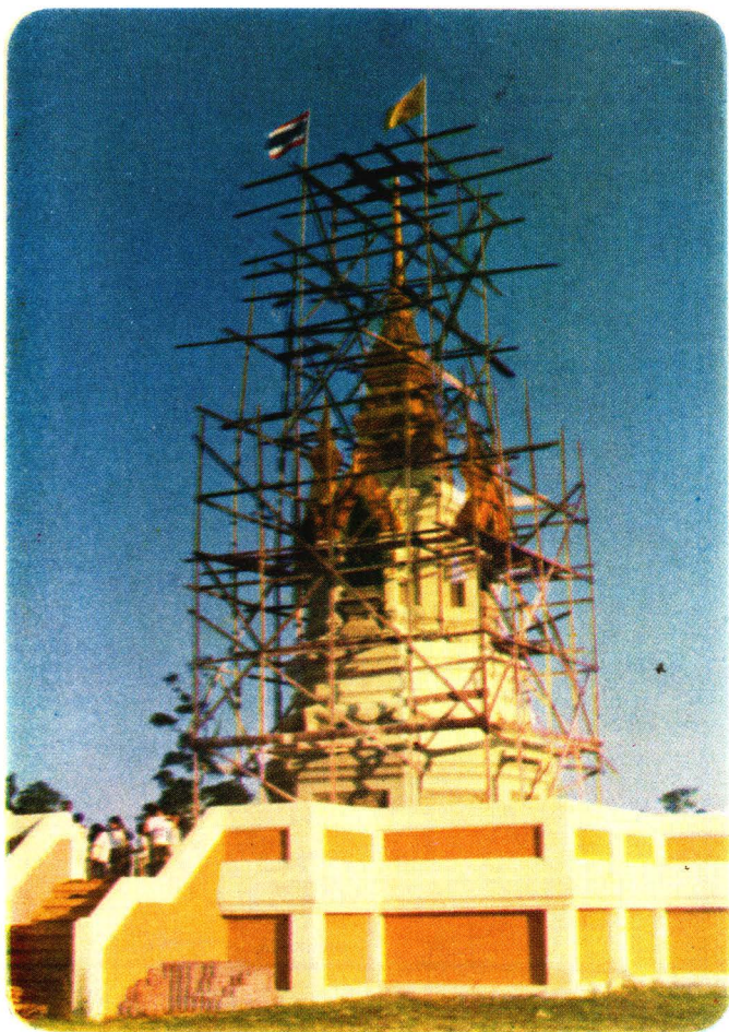
The Freedom Pagoda under construction within the Pine Camp, Petchaboon Province, Thailand
